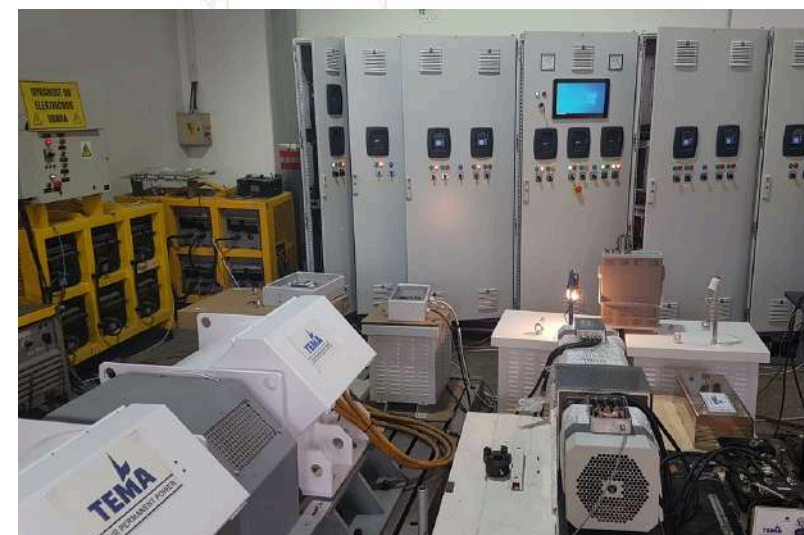
During FAT and DNV commissioning
